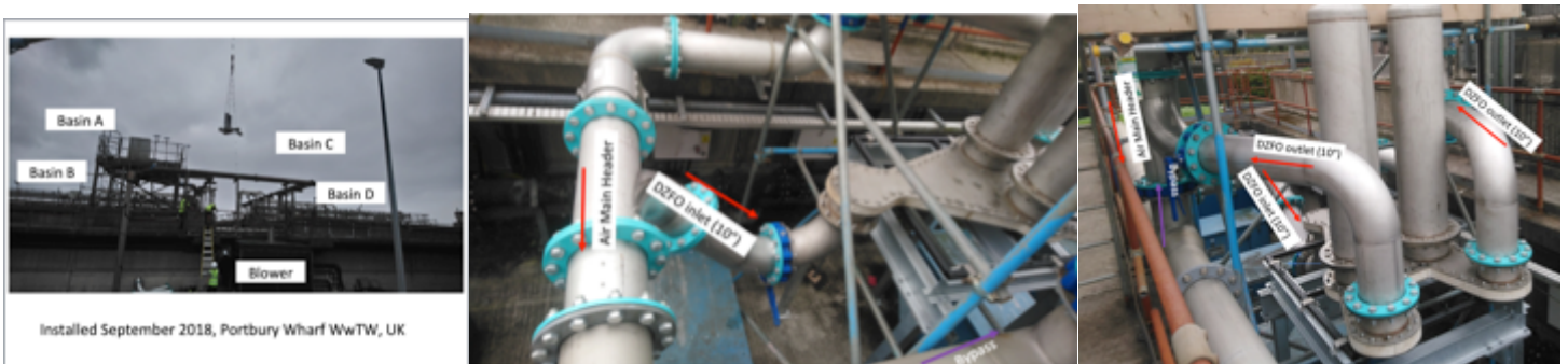
Figure 2 Installation of the DZFO on site- Retrofit installation as a valve in between blower and sparger to switch the gas.
