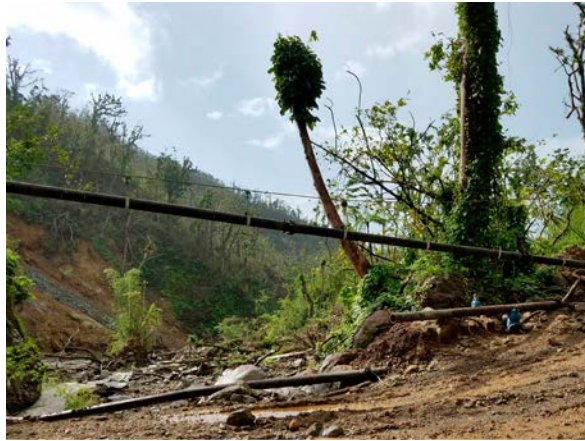
Water infrastructure highly exposed to landslides and flooding in Dominica. Images courtesy of DOWASCO
