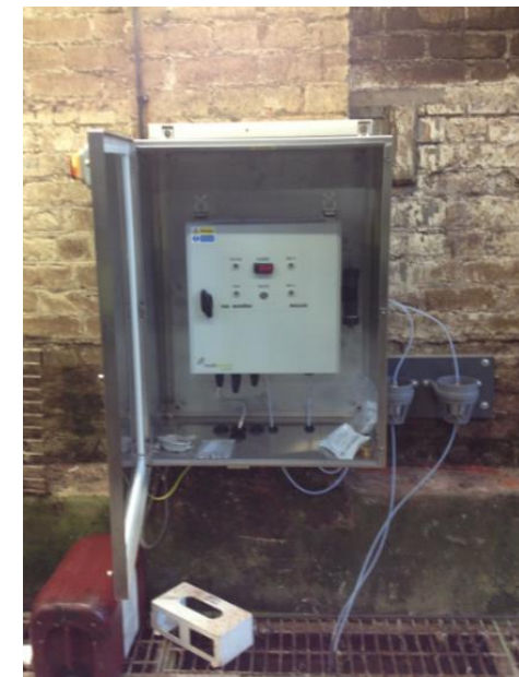
Unit installed in a wastewater plant in Scotland to detect high levels of VOCs
