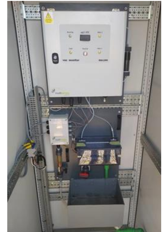
A picture of the unit installed in the outbuilding.
