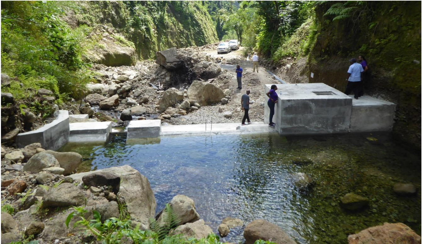
Water intake in Dominica under reconstruction using a more resilient design in following its destruction during flooding caused by Hurricane Maria in 2018.
